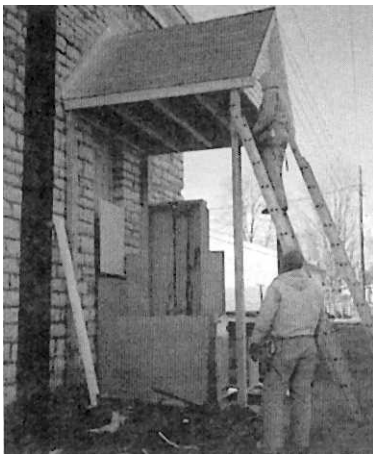
Covering an exterior liftbox protects it from weather.
